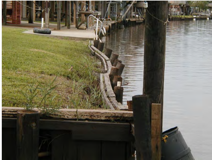
BH2—Class 4 Still Structurally Sound, Fill Maintained, Yet only in Average to Fair Condition.
