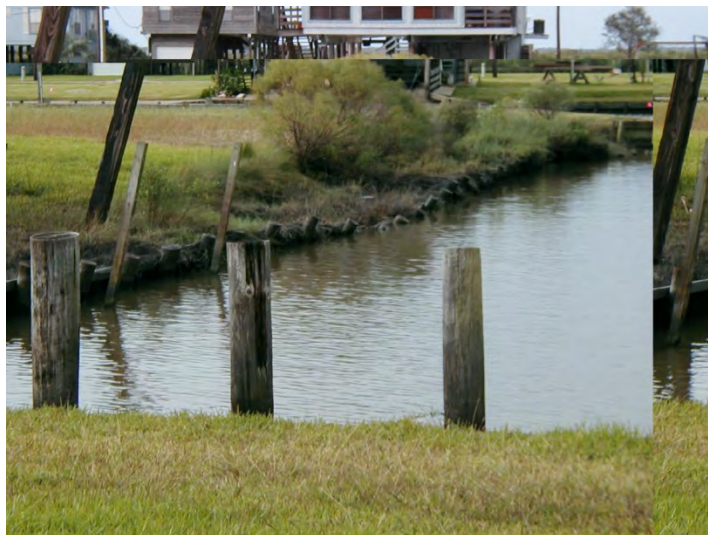
BH2—Class 4 Most of Bulkhead has given way, yet fill has been maintained. Fair to Poor.
